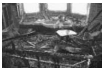
View of the fourth floor rear, where the fire began.
