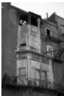
View of the north side of the main house after the fire.
